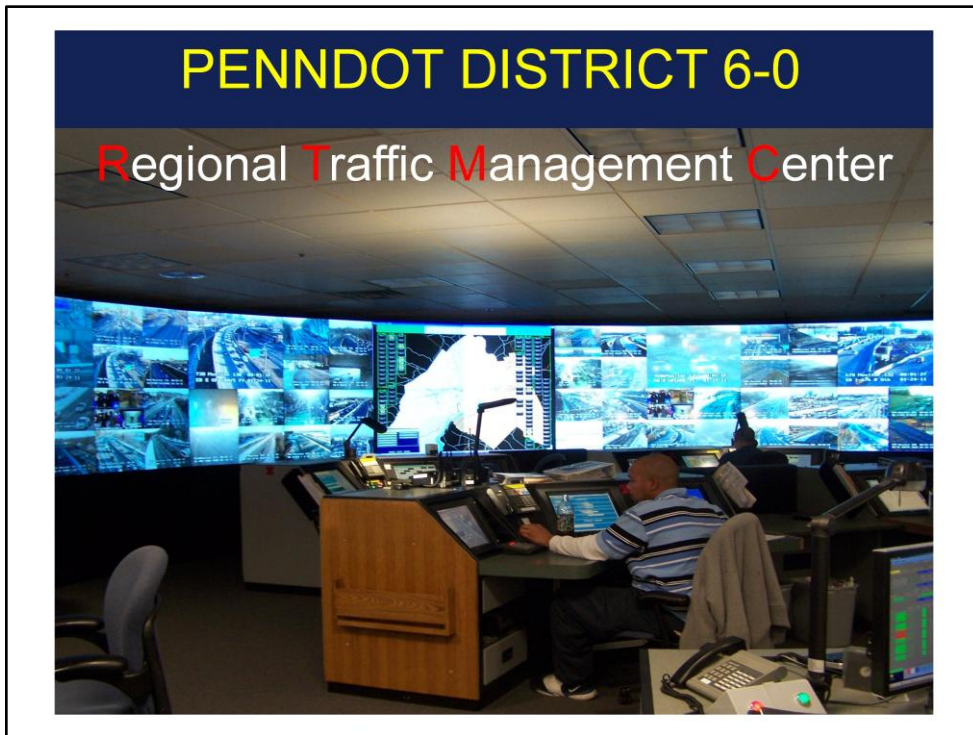
This is a view of the District 6-0 RTMC operations floor. The wall is comprised of 20 – 50” Mitsubishi cubes and the floor accommodates 6 work stations.
